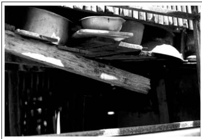
A broken joist beneath a kitchen
