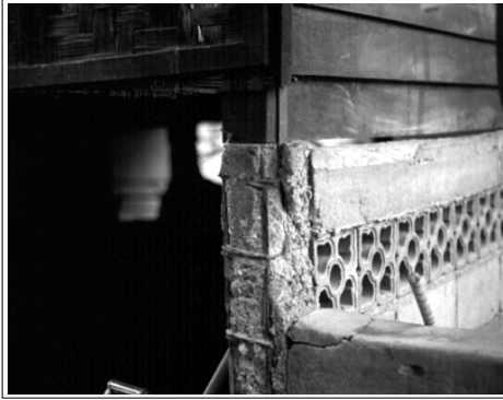
Failing reinforced concrete post
